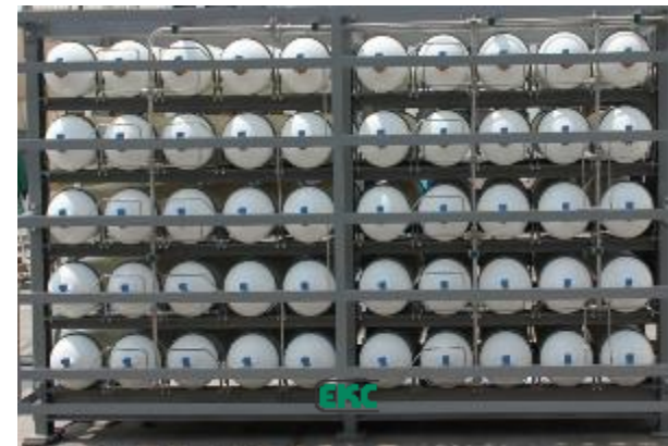
CYLINDER BUNDLES/ RACKS
