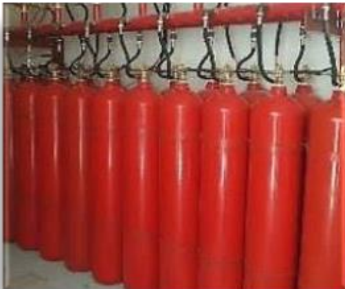
FIRE SUPPRESSION SYSTEM
